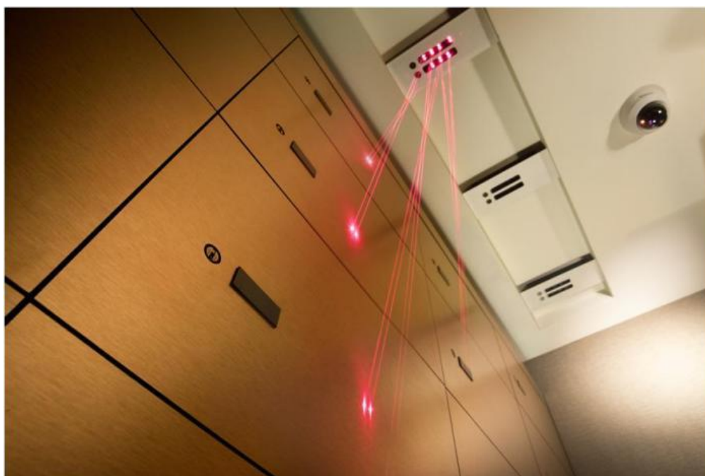
The Royal England vault is equipped with Special Lighting System to indicate the position of each safe deposit box rather than conventional numbering system
